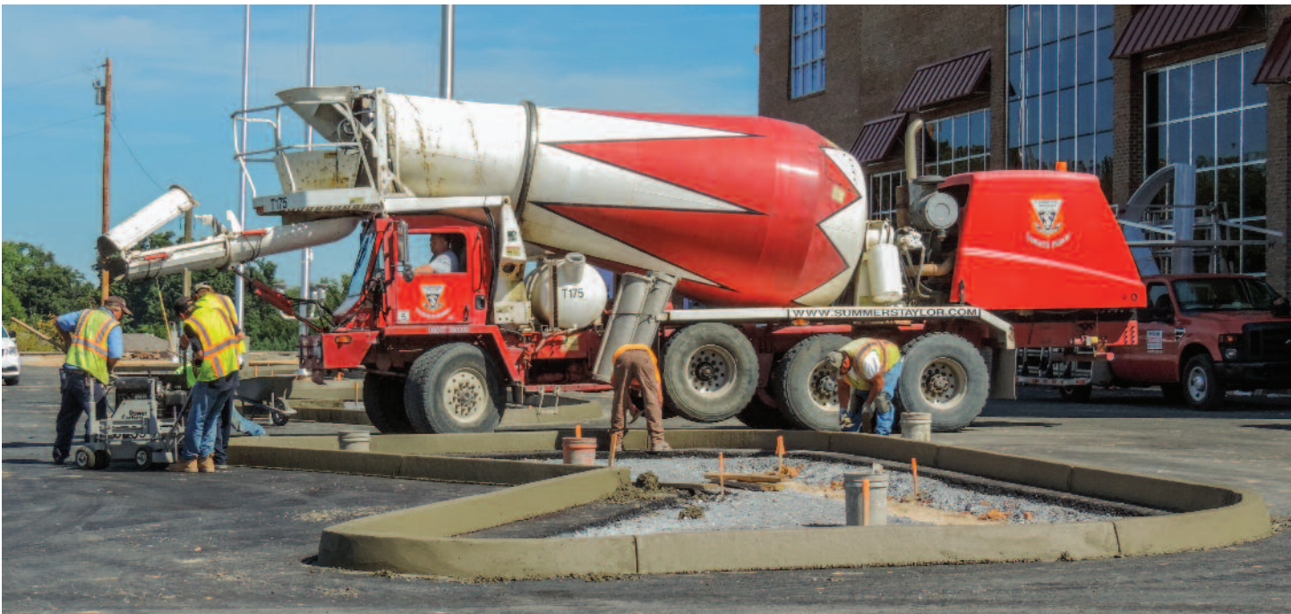
For jobs that require less expensive scab-on curb, extruded curb can be the ideal solution.
