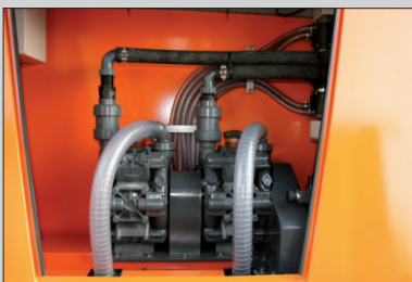
Logically designed liquid system with diaphragm pump.
