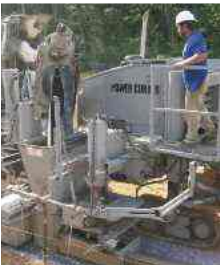
Operator has great visibility of entire process.
