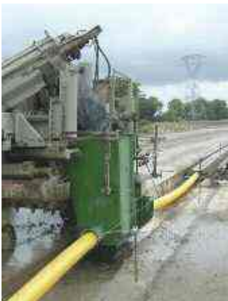
Slotted drain in Uzbekistan showing inflated tube.
